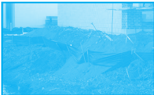
Failing silt fence. Photo courtesy of City of Toledo, Environmental Services.
